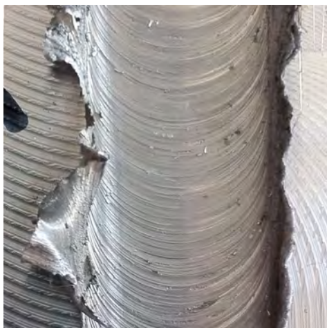
(a) Poor weld surface condition
