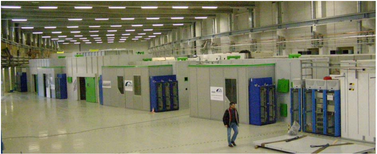
Figure 1: Experimental hutches and control cabins of the HEMS beamline at PETRA III.
